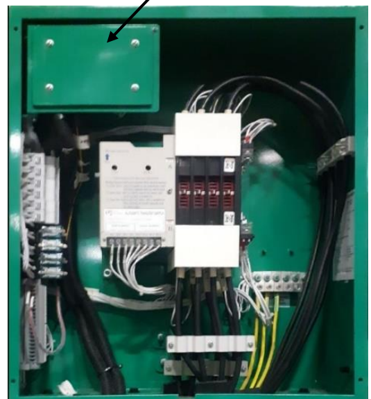
ATS with PowerStart 0600 controller
